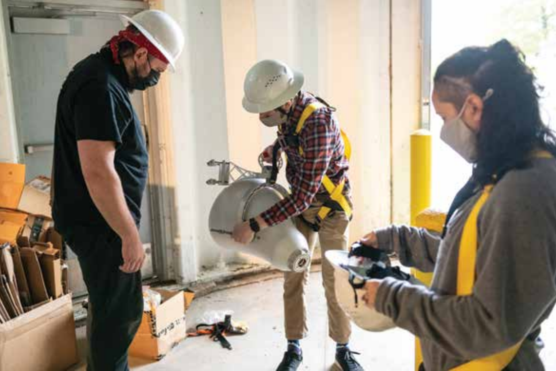
Sam Garfinkel (DC 2020), far right, and Meta Mesh team members installing Wi-Fi equipment at the water tower in Coraopolis.
